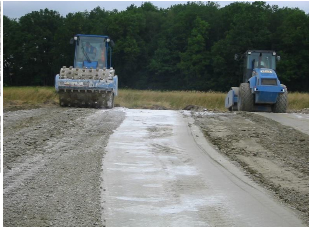
Compaction plant (VP5 and V5)
